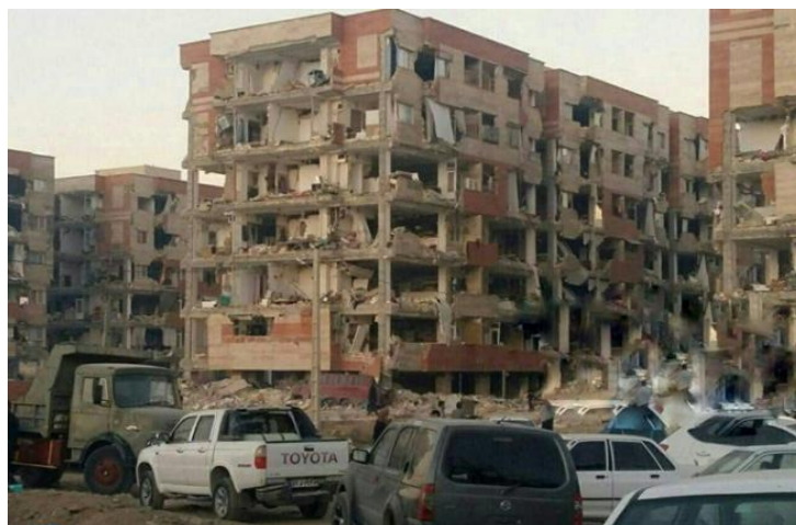
Fig. 1. Damage to infill walls during the 2017 Kermanshah earthquake.
