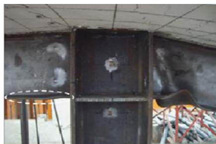
Fig. 8. Cracks in the slab in the middle connection area.
