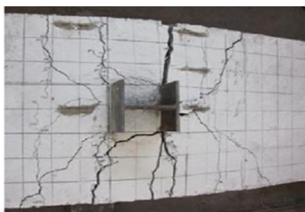
Fig. 10. Cracks in the slab at connection area B.
