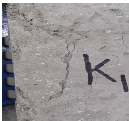
Fig. 12. Cracking in a sample without fibers.
