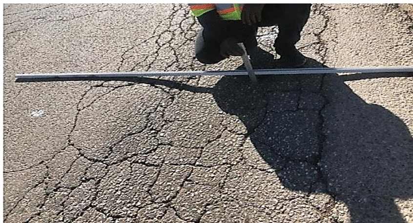
Fig. 7. Road pavement rut detection [59].
